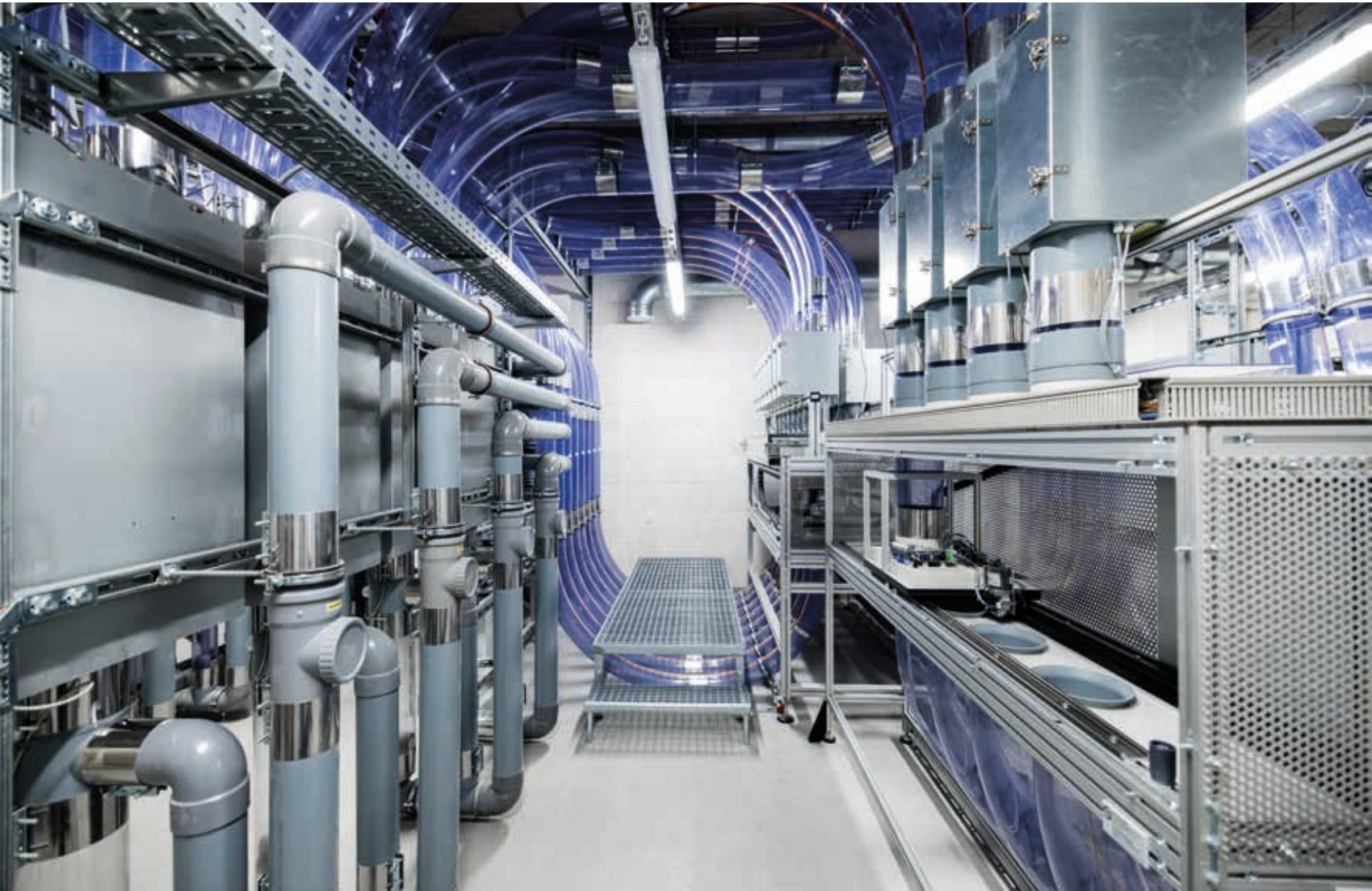
The installation of transparent tubes and bends gives the system a unique, almost artistic character.
